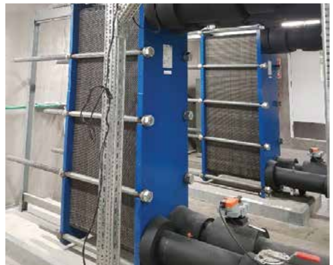
Heat exchangers for a groundwater sourced heat pump system.
